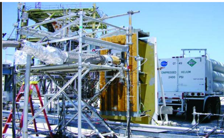
Testing of gaseous hydrogen vent arm umbilical disconnect equipment at Kennedy Space Center.
