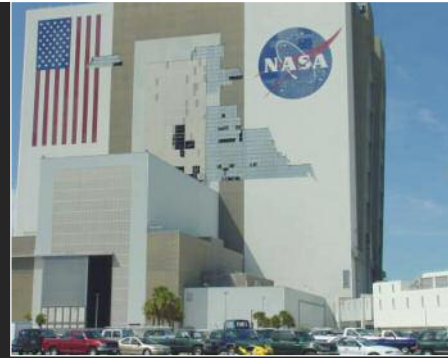
Damage to Vehicle Assembly Building at Kennedy Space Center during Hurricane Frances.
