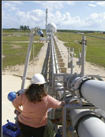
Hydrogen-sensing tape application at liquid hydrogen cross-country vent line flanges on the pad slope.
